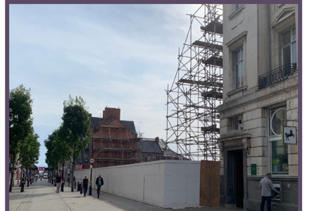
View east along King Street with cleared buildings where the new TCCC will be located
